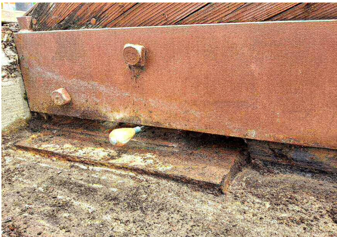
Description: Rotting of timber member at bearing - north end, downstream side
