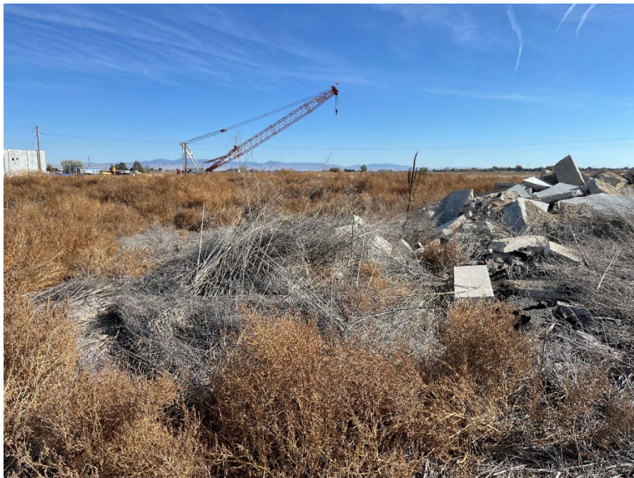
Photograph 6. Concrete debris pile near old lateral location
