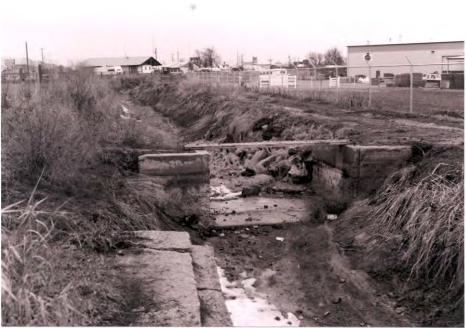
February 2, 2001 photograph of Canyon Hill Lateral to the northwest showing abutment, headgate and encroaching development
